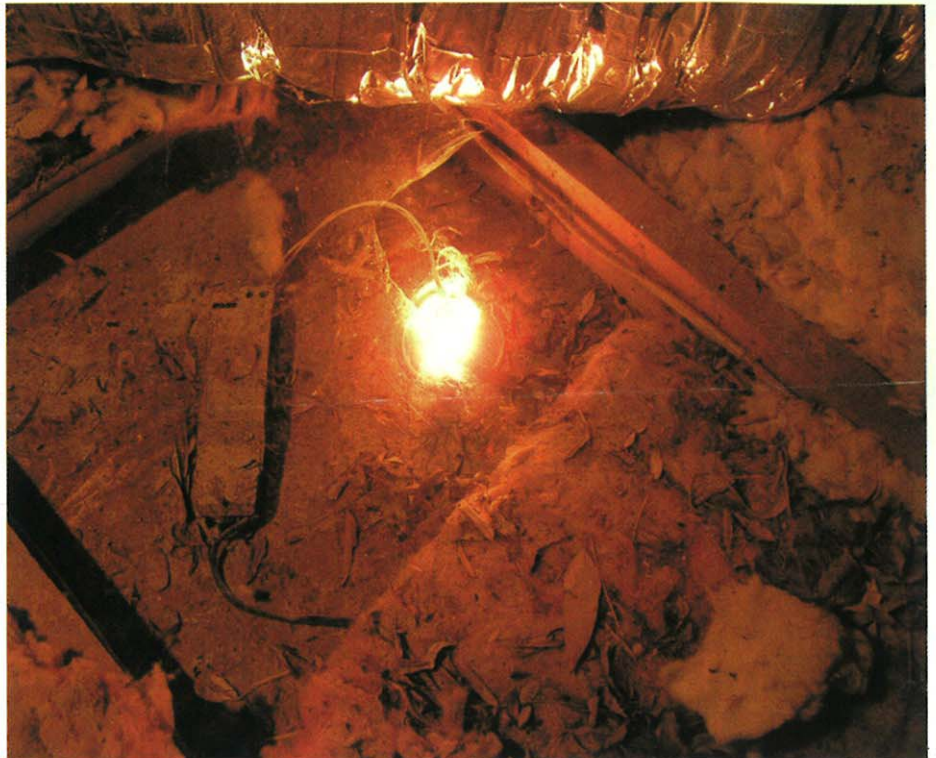
The first changes to the Wiring Rules in seven years means builders must be aware of how they too can be liable for the faulty installation of downlights and take steps to protect their businesses.
